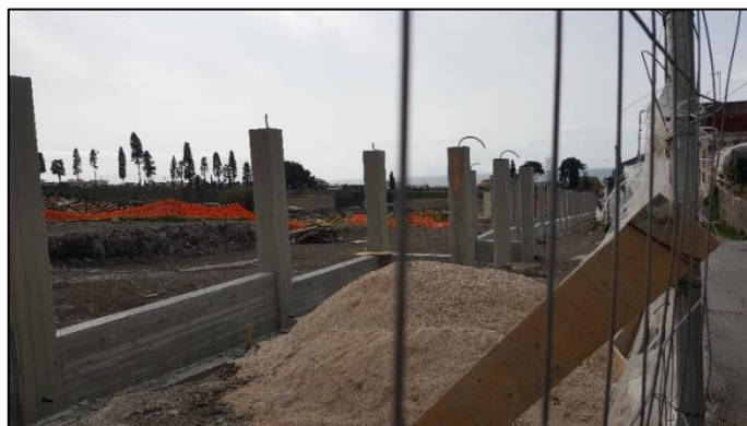
Figure 8. 13. The boundary wall between the archaeological site of Herculaneum and the Via Mare neighbourhood until 2019 (above), the proposed new boundary that will substitute it (middle) and the construction work of the new boundary wall in 2020 (below) (Resource: Studio Barbieri; Negri/ HCP, cited in Court et al., 2019: 30; Personal archive, 2020)
