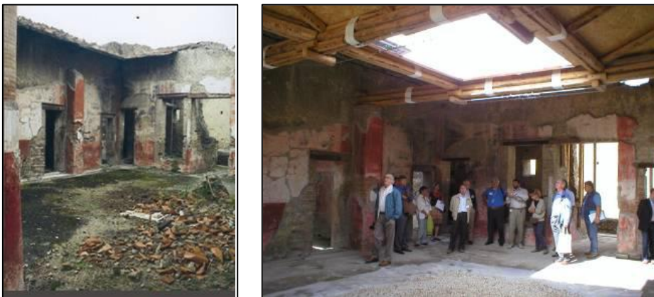
Figure 8. 3. The atrium of the ‘House of the Gem’ before and after emergency measures and the installation of a medium-term roof (Resource: Jane Thompson/ HCP, cited in Thompson, 2007: 5)
