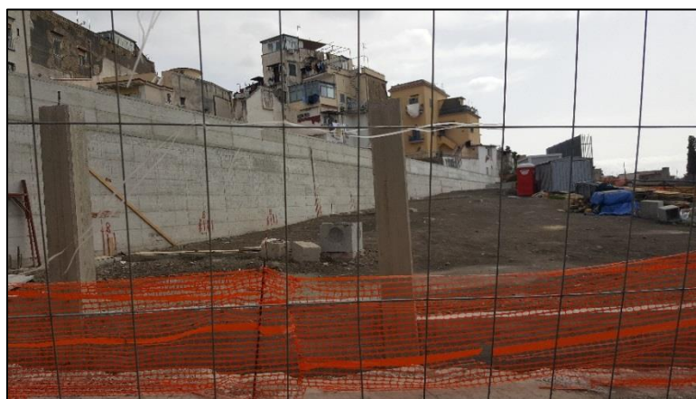
Figure 8. 12. The new boundary wall and the new park and square being constructed between the archaeological site of Herculaneum and the Via Mare neighbourhood on the abandoned lot (Resource: Personal archive, 2020)
