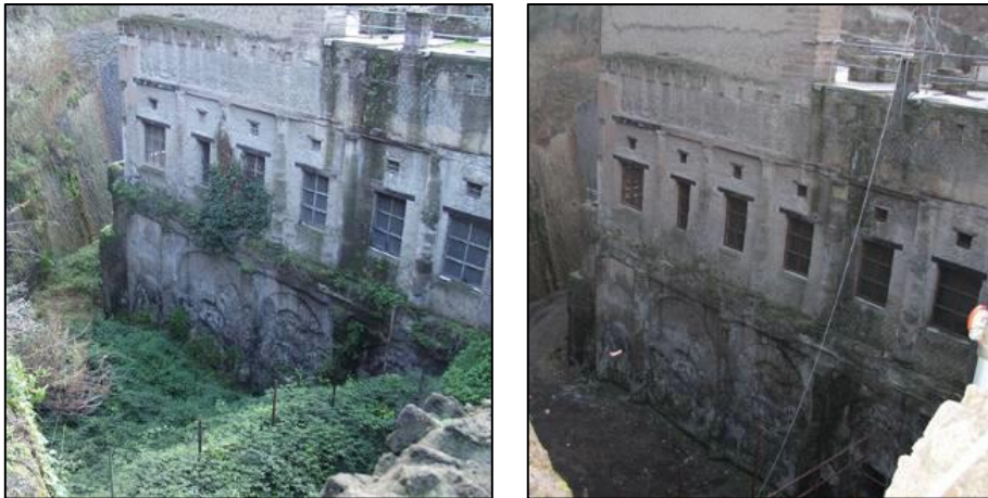
Figure 8. 2. The ancient shoreline and the facade of the ‘House of the Telephus Relief’ before and after the removal of vegetation and the installation of pigeon nets (Resource: Paola Pesaresi/ HCP, cited in Thompson, 2007: 5)
