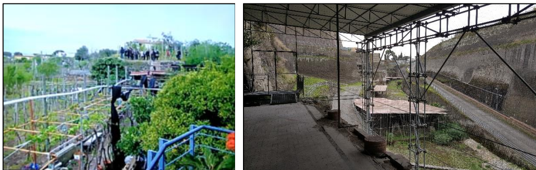
Figure 7. 23. The expropriated area before excavation (left) and after excavation (right) (Resource: Project Manager; Personal archive, 2020)
